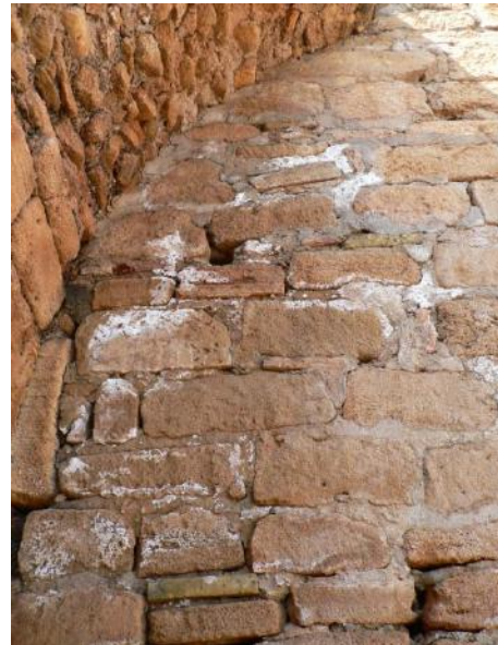
Fig. 4: Damage Salt develops as encrustation covering the stone in interface with cement mortar
