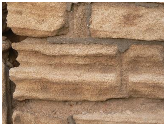
Fig.8: In contact with cement mortar, the rock has deep grooves that hollow out the material highlighting the hardest levels
