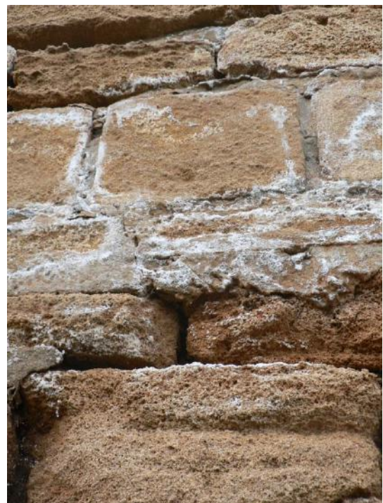
Fig. 5: Details of the saline efflorescences and encrusting on the calcarenite of Salé, at the interface stone-mortar
