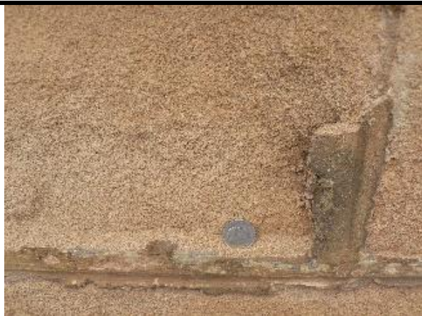
Fig. 6: Granular decomposition of a block of calcarenite, consequence of the use of a hard cement mortar. The rock has grown into a single alveolus.
